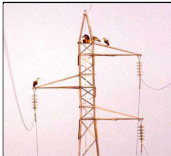
Figure 3: Curicacas perched on metallic tower of 69 kV TL [5]
