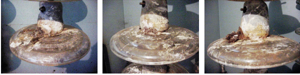
Figure 9: Insulators removed from service [7]
