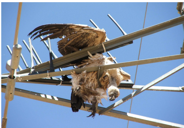
Figure 1: An electrocuted vulture on an 88 kV steel lattice structure (photograph courtesy of Johan van Staden)
