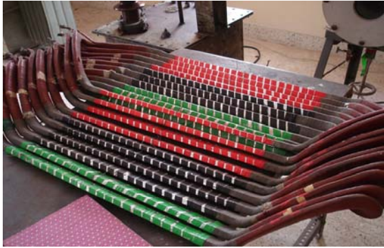
Figure 7: A view of motor stator coils under test
