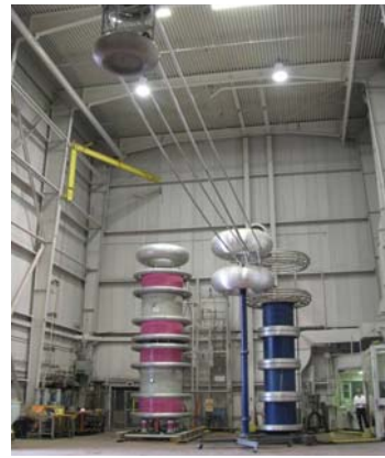
Figure 1: Setup of the positive pole of the bipolar dc transmission line
