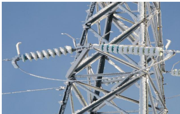
Figure 17: Ice accretion on glass insulators on adjacent towers
