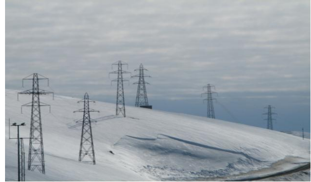
Figure 3: Decommissioned line on high altitude trial site
