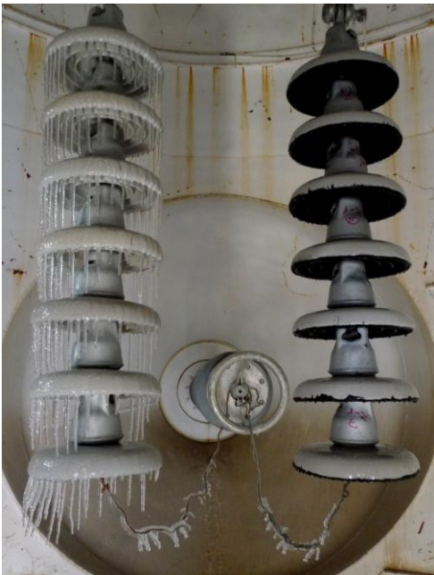
Figure 3: Icing on clean surface
