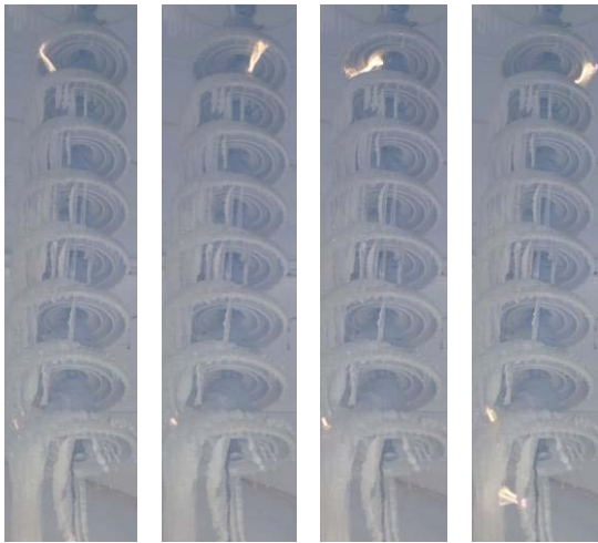
Figure 4. Discharge of the insulator strings. Photos were taken at the sixth hour when the discharge is serious.
