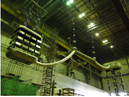
Figure 1, Valve Module attached to the DC test supply
