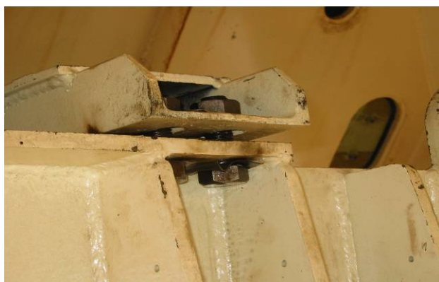
Figure 5: strong looseness in the core of transformer
