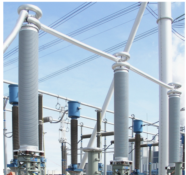
Figure 11: PD-free test set-up for 380 kV resonant test of three phases in parallel
