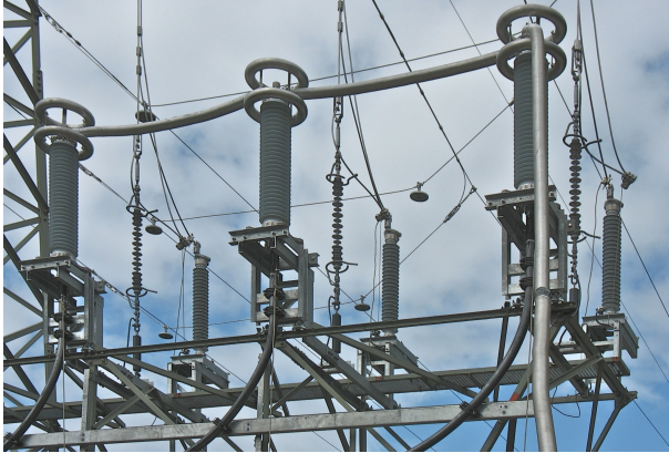
Figure 2: PD-free test set-up for 160 kV resonant test of three phases in parallel
