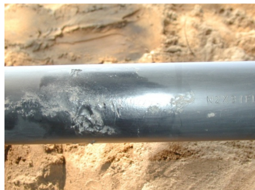
Figure 3: Cable sheath damage after breakdown at a 110 kV-cable
