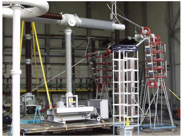
Figure 10: Example of a making test on a 245 kV CB (middle) with spark path tower (right) and charging unit (middle right) and voltage divider (left)
