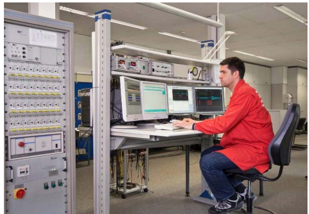
Figure 11: Control and measurement room of the high-power laboratory
