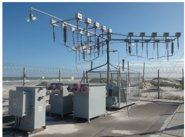
Figure 1: AC / DC insulator test rig
