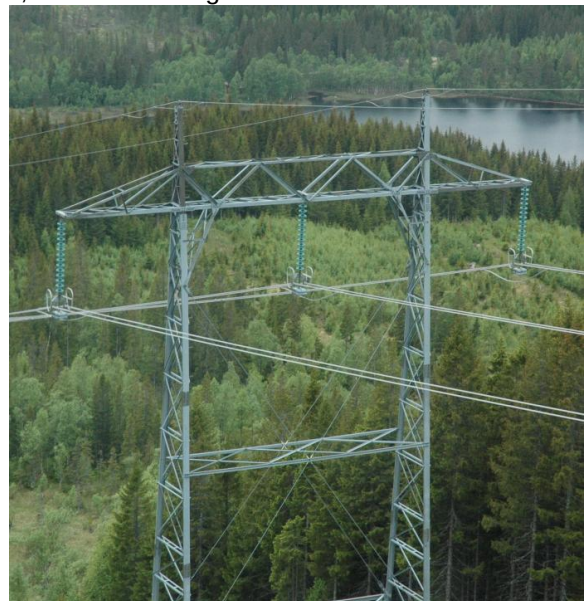
Figure 1 Showing a suspension tower in 300 kV, duplex line (picture comes from [4])
