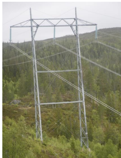
Figure 1. A typical 300 kV tower with duplex arrangement and single I-strings before upgrading.
