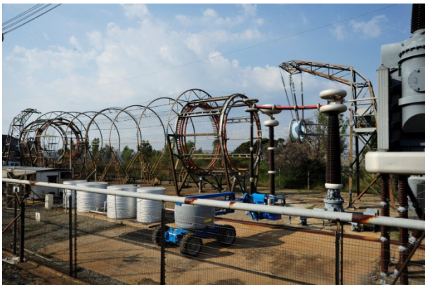
Figure 2: Lateral view of the Eskom Corona Cage.
